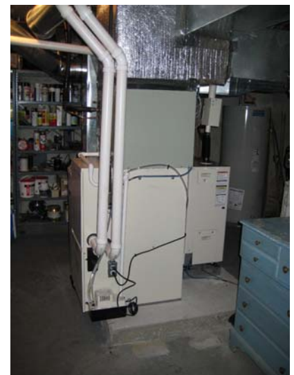
Warm Air freewatt System #1 (Side View)
