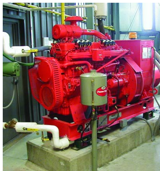
Northern custom designed this propane-fueled, combined heat and power system for Green Mountain Coffee Roasters.
