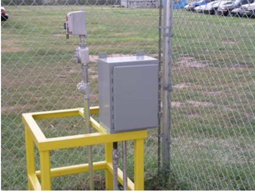
Remote meter and conditioner for cells
