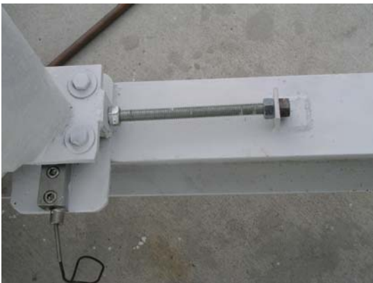
Load cell installation at the foot of the tank. Four load cells were installed.
