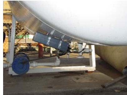
Picture 6: Installed Beta 1.1 Prototype
