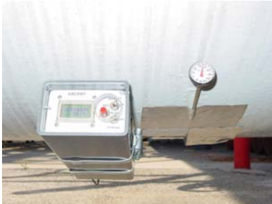
Picture 5: Installed Beta 1.1 Prototype
