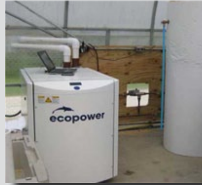
A Marathon Ecopower propane-fueled CHP system is being demonstrated in a Pennsylvania greenhouse.
