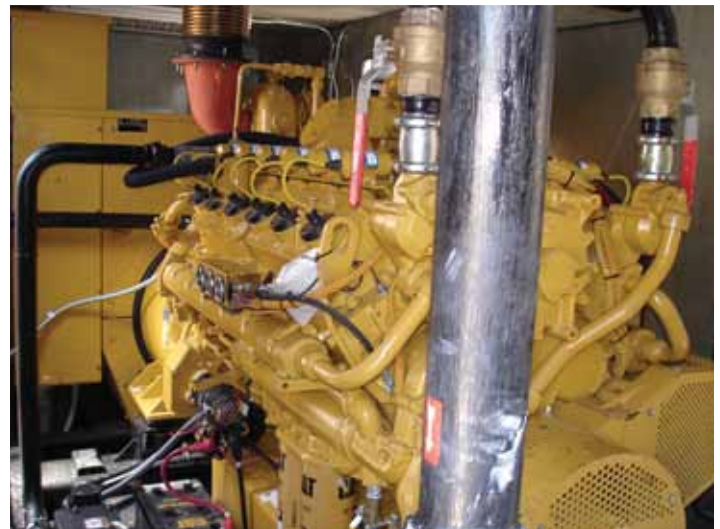
The three-phase, 405-kilowatt Caterpillar generators are rated at 506 kilovolt-amperes, 480 volts, 1,800 revolutions per minute, and 60 Hertz.
