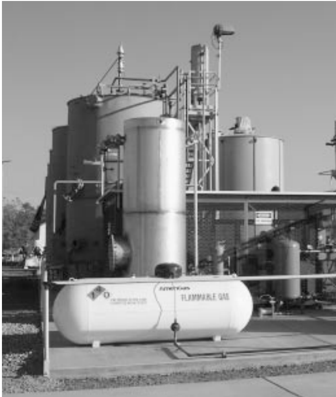
Biogas Energy Project at UC Davis
