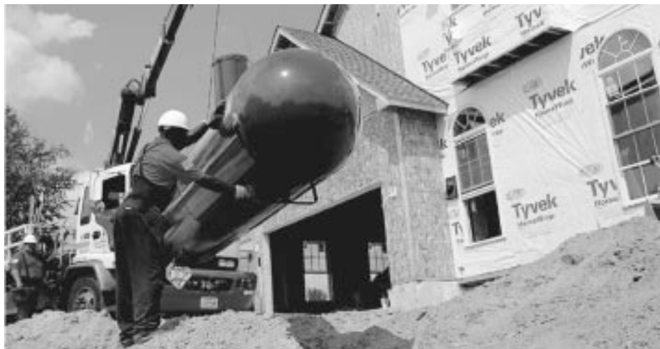
This underground tank picture was used in builder ads that ran in Custom Home , Builder News , and Custom Builder .
